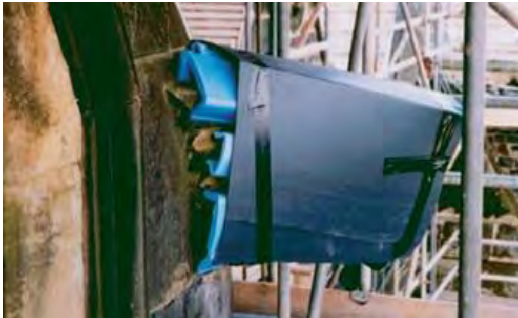
Figure 2 A gargoyle at Grey Towers, Nunthorpe, well wrapped in U-profile foam protectors and TwinShield to protect it from traffic along the scaffold
